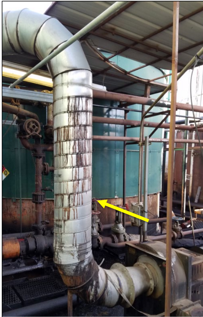
Figure 2: VPC Inlet Ductwork
